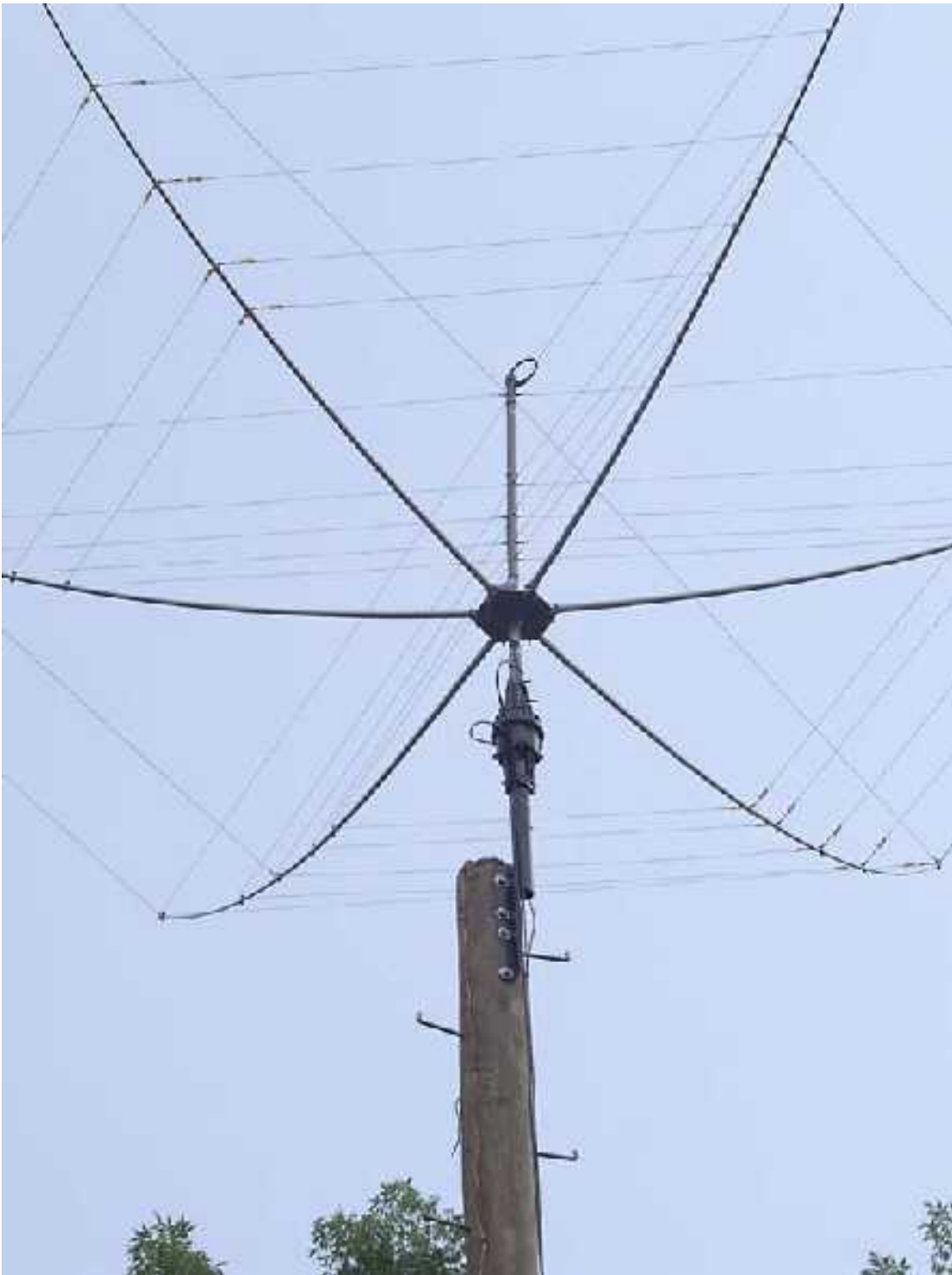
Here is a detailed picture of the completed rigging of the feedline for the HX-5Bi HexBeam, and the control cable for the Yaesu G-800SA rotator. Proper strain relief for the cable is the next step to be done.
